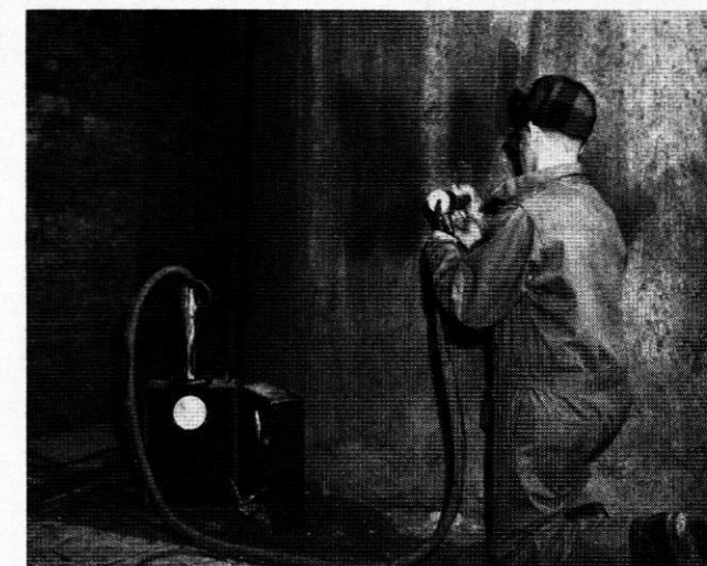
An engineer takes an electrostatic precipitator sample in a stack of the steel mill.
