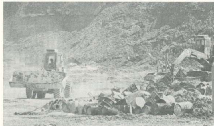
Equipment contaminated by PCBs in the Emelle landfill. (Phil Scarsbrook)
